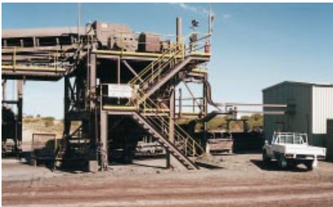
Conveyor plant drive unit
